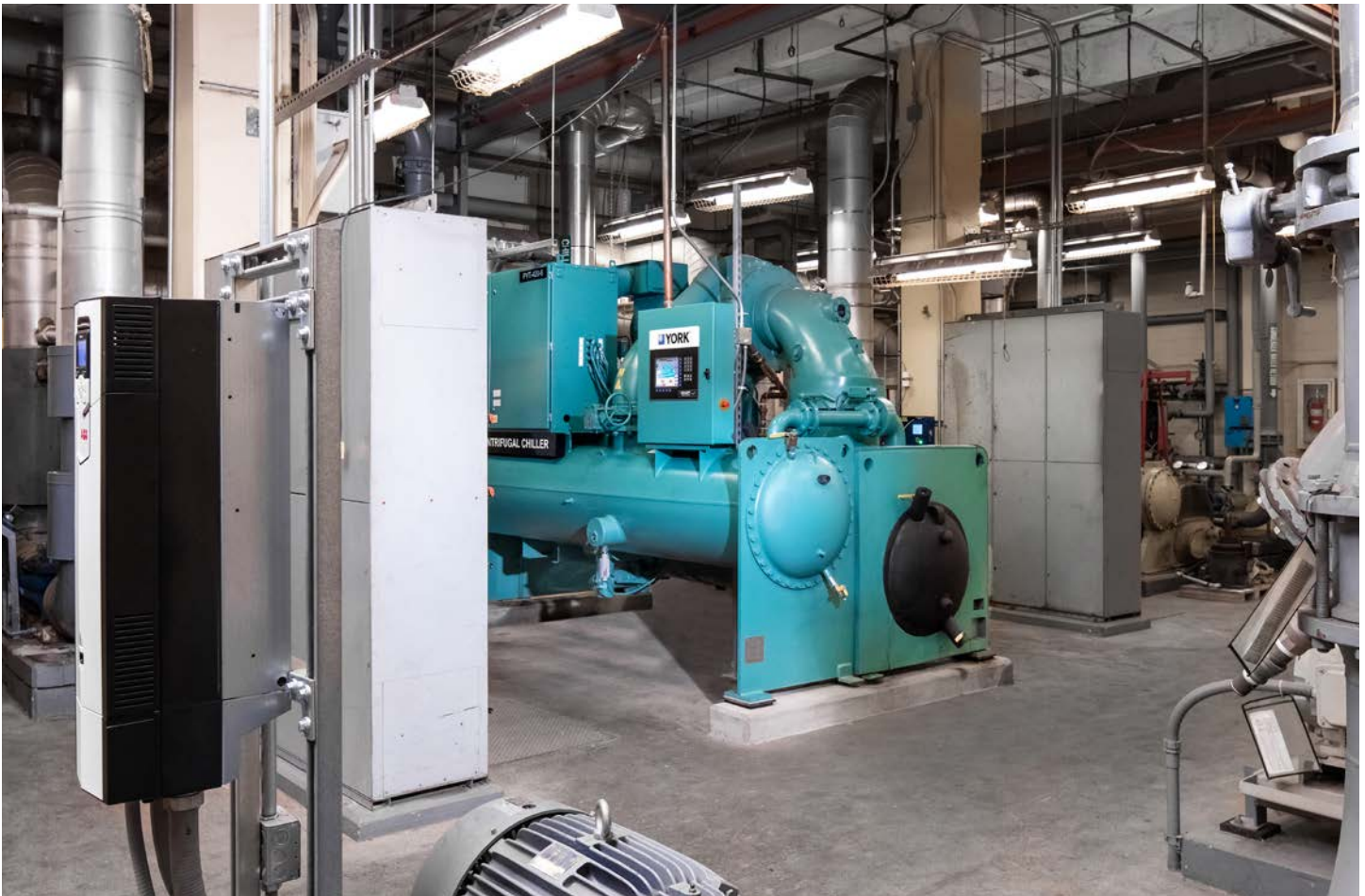
The 300 ton YORK® YZ Magnetic Bearing Centrifugal Chiller replaced two older chillers in the Pickle Research Center
